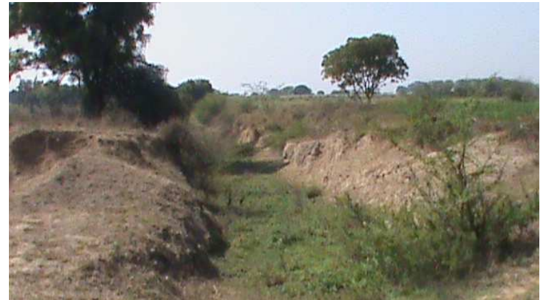
Fig. 3.3: Severe erosion in the watershed
